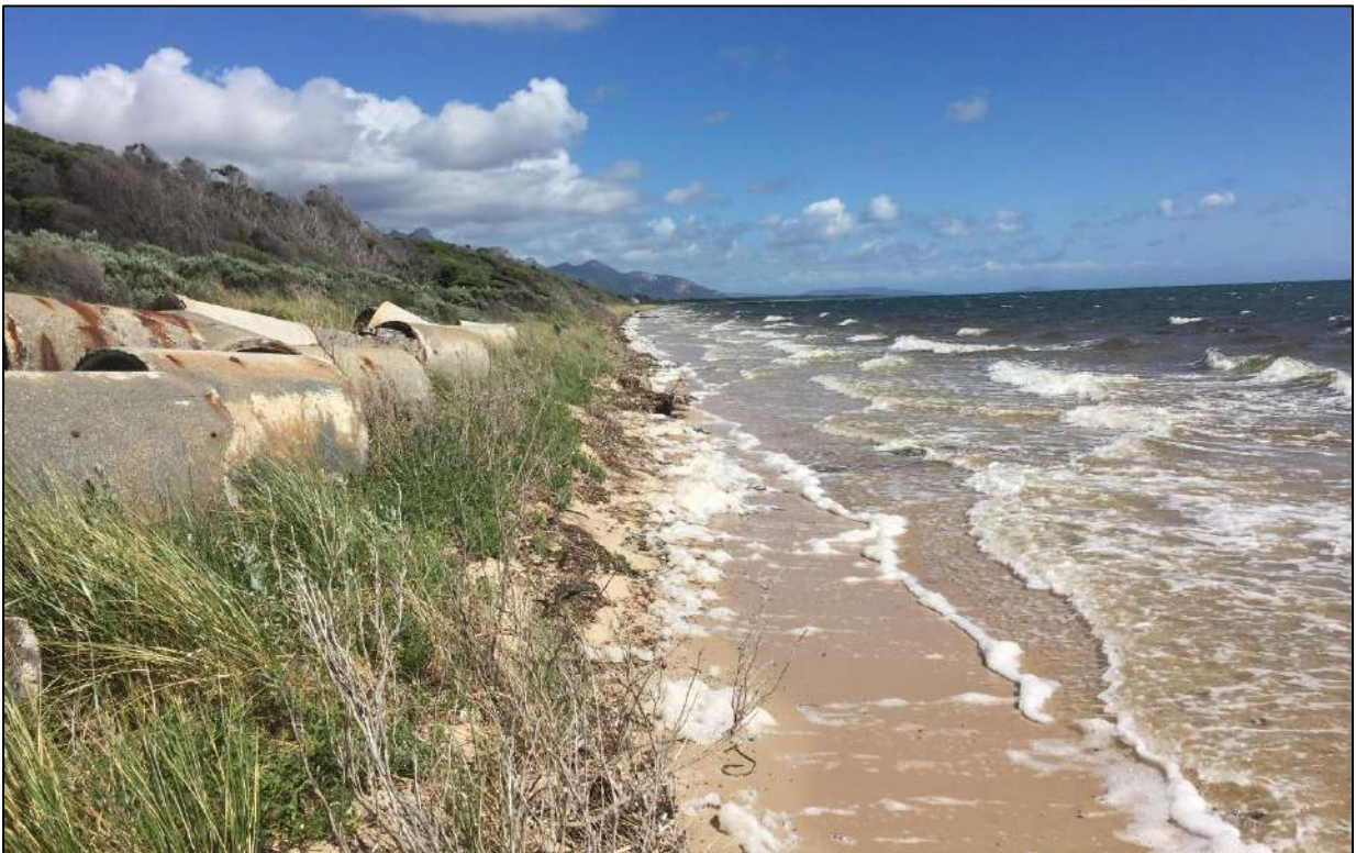
Plate 7 Damaged storm water pipe sections which drain the northern (Hayes Hill) catchment were displaced in the recent storm. Regular and combined influence of high tide, wind setup and wave runup is actively scouring fine grained sand on Whitemark Beach ~1km to the north of Whitemark.
